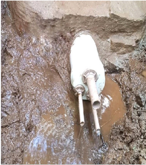
2A - kit Sanear instalado
